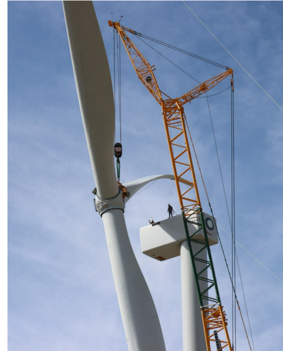
Installation of the final wind turbine at PSE's Beaver Creek wind farm in Stillwater County, Montana in Sep. 2024.
